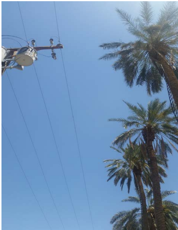
Exhibit 4. The proximity of the power lines to the palm trees.
