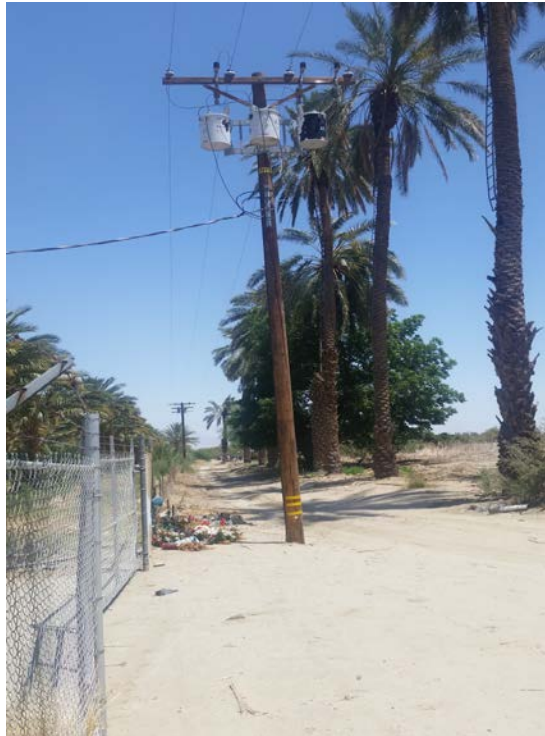
Exhibit 3. Location of truck (adjacent to power lines).
