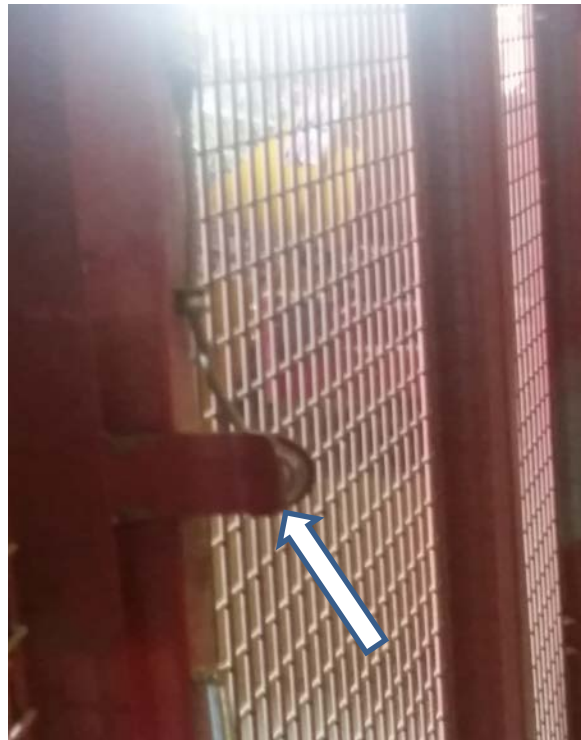
Exhibit 9. The safety sensor on the gate.
