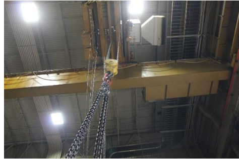
Figure 3. Bridge crane on site.
