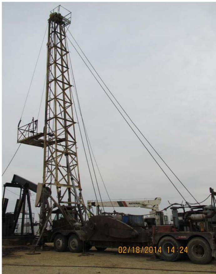
Exhibit 3. The rig at the incident scene with the boom extended.
