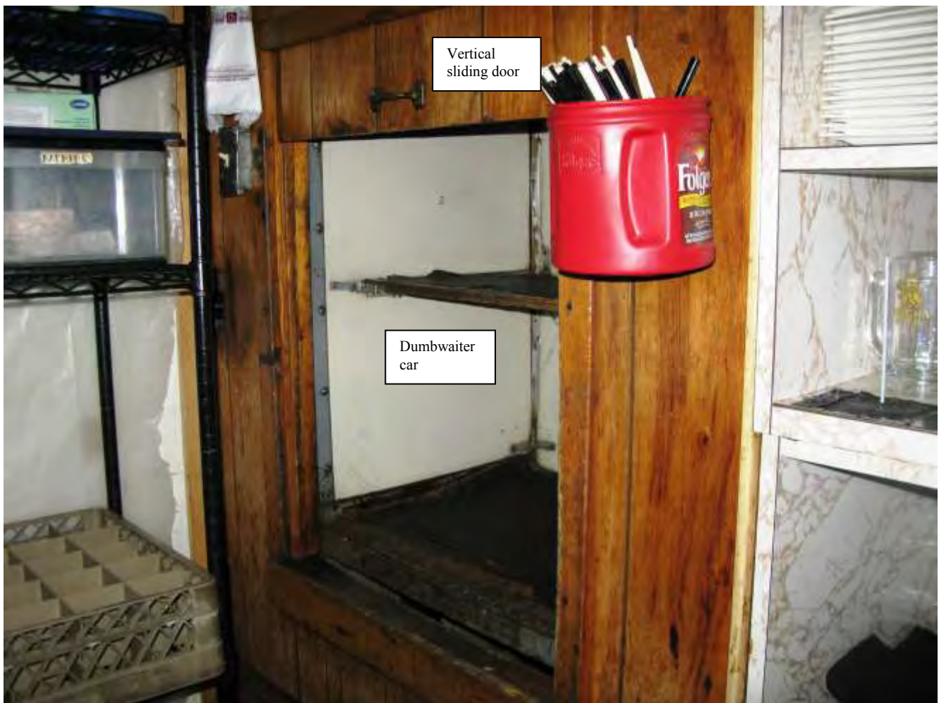
Photo 1. The hoistway door opening in the upstairs food preparation area with the dumbwaiter car in the landing zone. The sliding door was nailed to stay in the up and open position.
