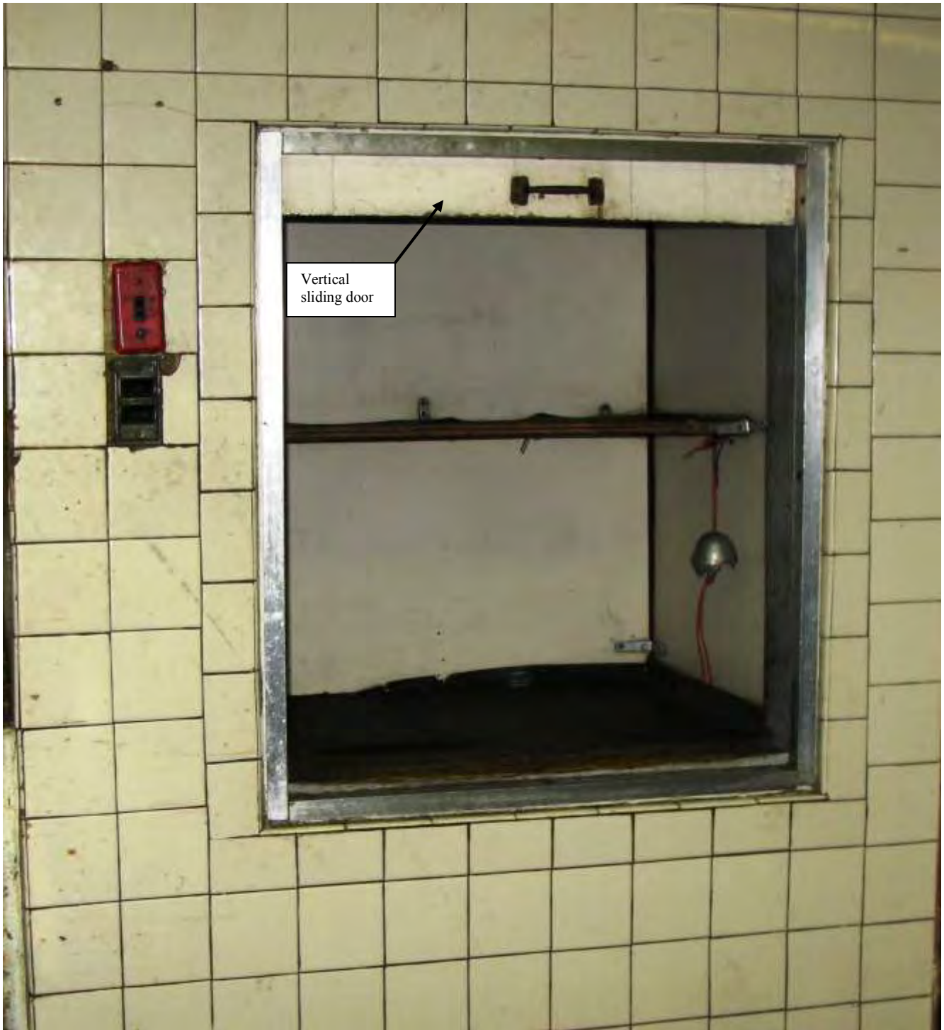
Photo 2. The dumbwaiter hoistway door opening in the basement kitchen with the dumbwaiter car in the landing zone. There were two black press switches one for UP and one for DOWN and a red on/off power switch to the left of the opening. The bell attached to the rack in the car did not work.
