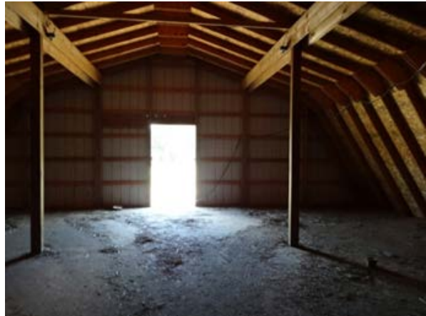
Figure 2. Standing in loft area, loft opening through which decedent fell
