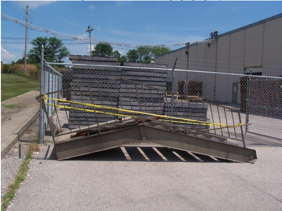
The metal stairway which had been attached to the building under the door. Laborer 1 was reported to take breaks under this structure. Photograph property of KY FACE
