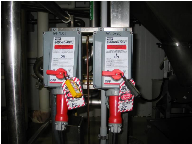
Figure 4 – The feed pump skid circuit shut off that is locked and tagged out after the incident
