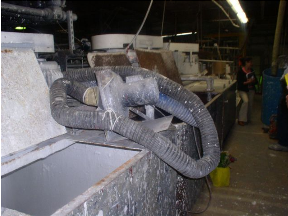
Exhibit 6. The air pump and hose that was used to remove contaminated air from the tank.
