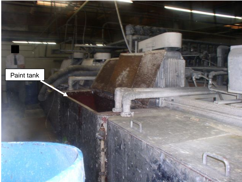
Exhibit 2. The paint tank the victim was cleaning.
