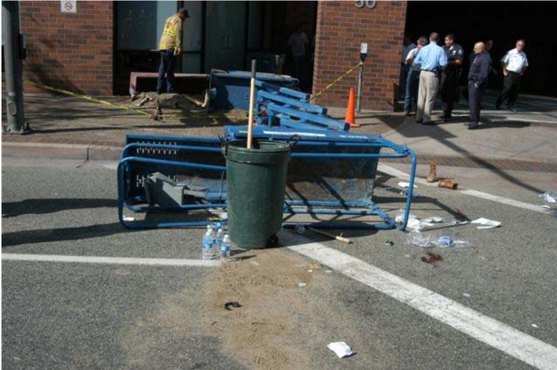
Exhibit 2. The work platform on the toppled scissor lift.
