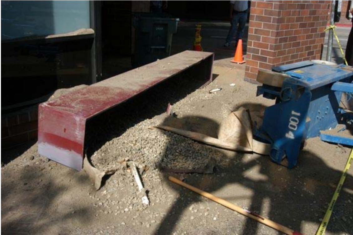
Exhibit 4. The planter box that knocked over the scissor lift.
