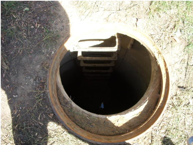
The incident sewer manhole was five feet in diameter and 18 feet deep with an opening 24 inches in diameter; the access rungs were sturdy and intact (Photo courtesy of NYSDOL-PESH).
