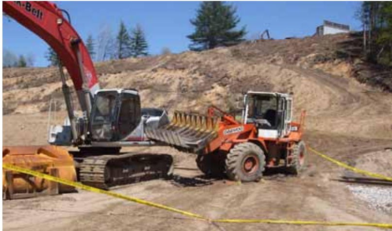
Figure 1. Overview of incident site
