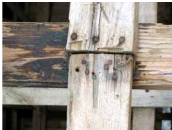
Figure 2. Fence board/post where some pilot holes had been drilled.
