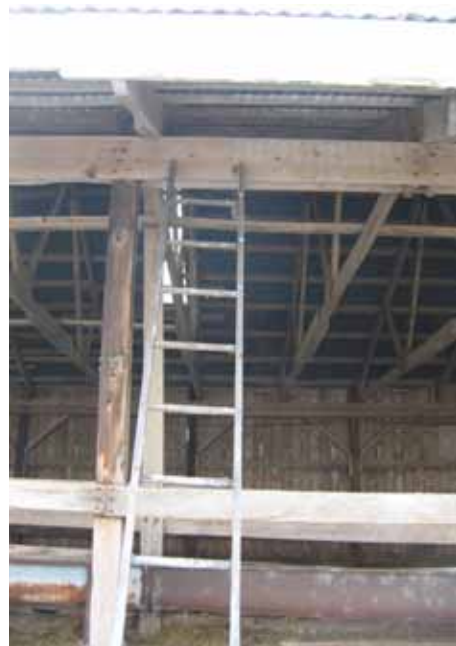
Figure 5. Top of ladder resting against the upper beam of barn
