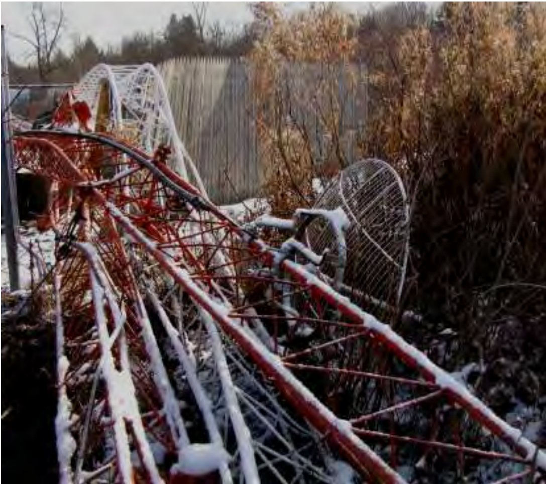
Photo 2. The collapsed communication tower (photo courtesy of OSHA).
