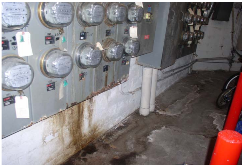
Exhibit #6. The water damage inside the apartment complex that warranted the waterproofing.
