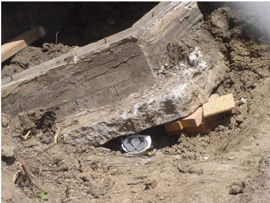
Exhibit #5. The concrete slab that fell on the victim.
