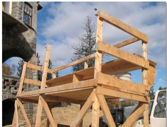
Photo 5 Upper Tier (courtesy of OSHA)
