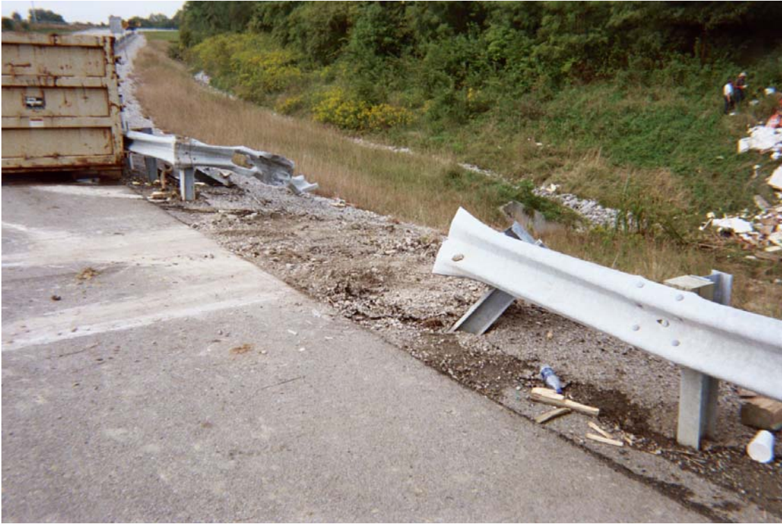
Area where semi went through guardrail.
