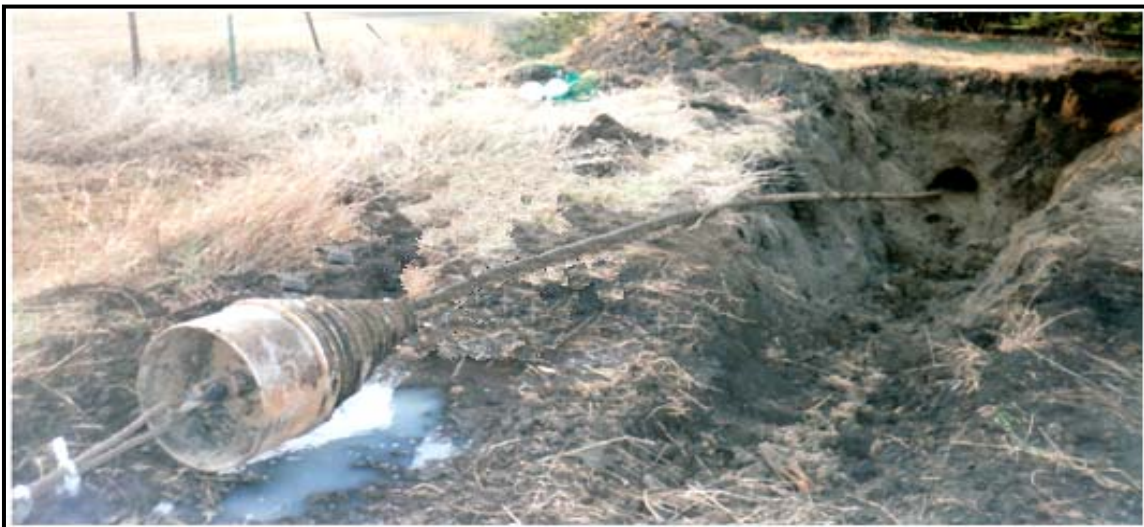
Photo 2 – Reamer connected to drill line at location where victim was found. Note arc in drill line and the reamer's position on the shoulder of the guide trench. Cable from reamer is connected to the pulling head secured to the pipe.
