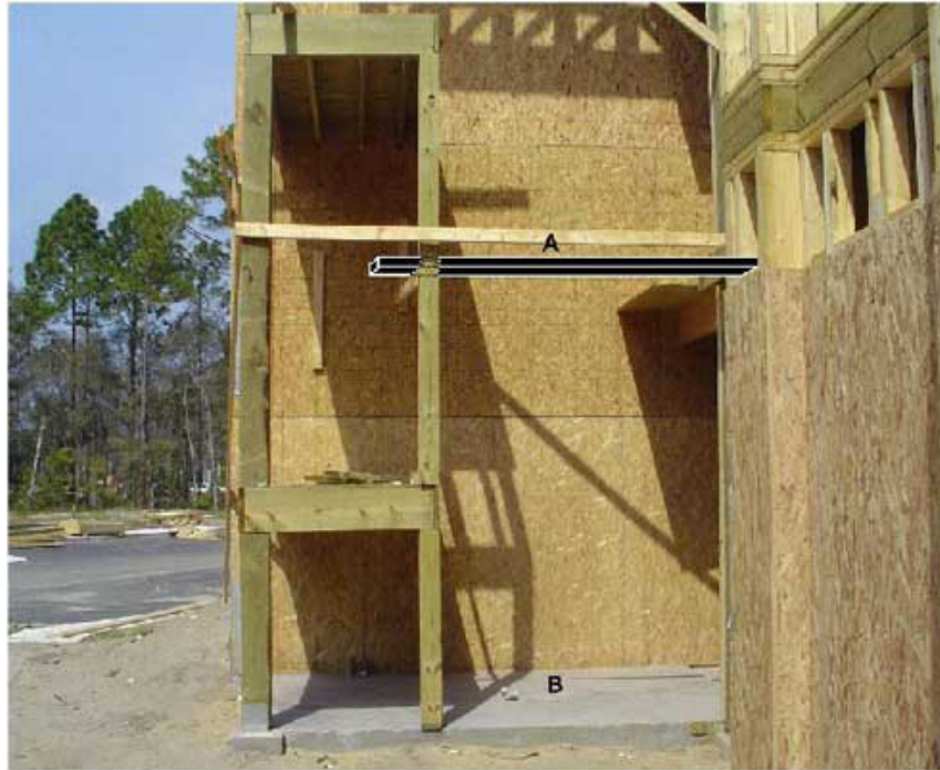
Photo 3 (Case Study 2). In this close-up view of the condominium stairwell and balcony area, the black rectangle illustrates the elevated platform, the letter A shows the young worker's approximate location before falling, and the letter B shows the approximate location of his fall onto concrete, about 10 feet below. Photo by County Coroner's Office, South Carolina
