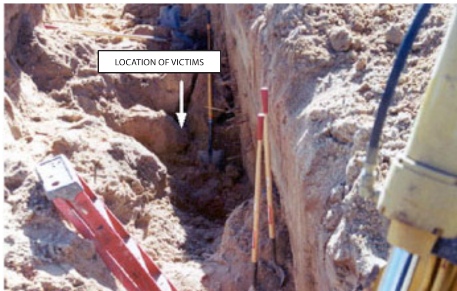
Photo 1 (Case Study 1). Location at which the two victims were buried by the trench collapse. Photo courtesy of county coroner.
