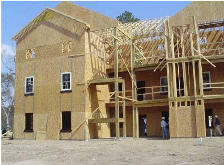
Photo 2 (Case Study 2). This condominium project was the site at which the worker's fatal fall occurred. Photo by SCOSHA.
