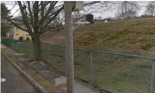
Figure 3 - One of the buckled sidewalk sections
