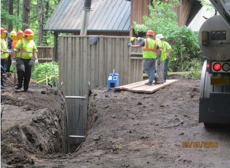
Figure 2. Emergency responders preparing to install a trench box before starting rescue and recovery work, to prevent risk of additional collapse and injuries
