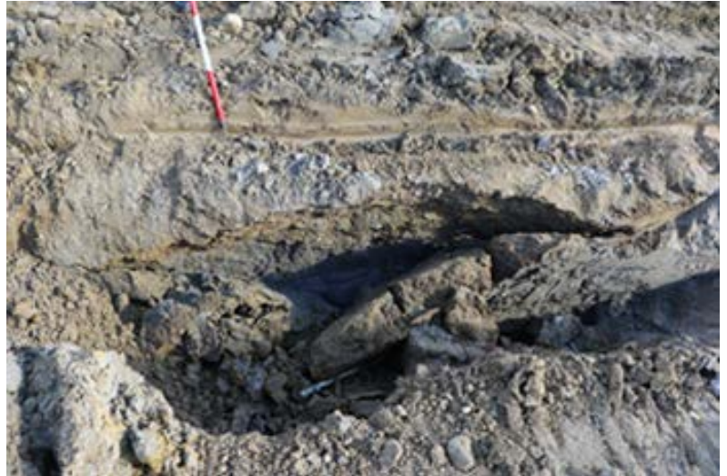
Figure 3. Trench wall collapse
