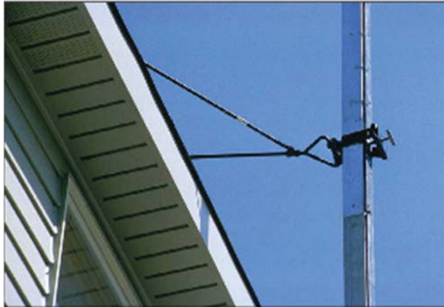
Figure 5. Example of scaffold pole properly secured to building (from OR-OSHA publication, "Supported Scaffolds").
