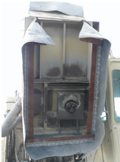
Figure 4. Installation of the air-blocking shelf at Mine A. The shelf is constructed of light gauge angle iron (silver) and thin, 63.5 mm, conveyor belting material (red).
