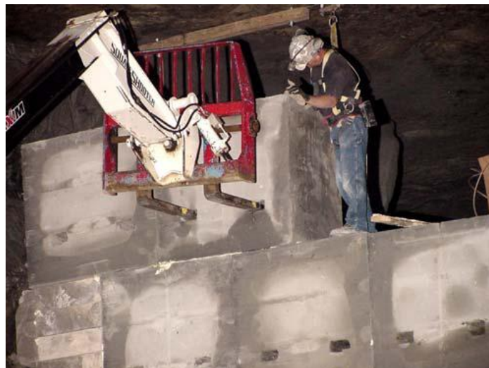
Figure 11. Omega Blocks used as a stopping for directing airflow. Picture courtesy of Grau and Meighen [2006].
