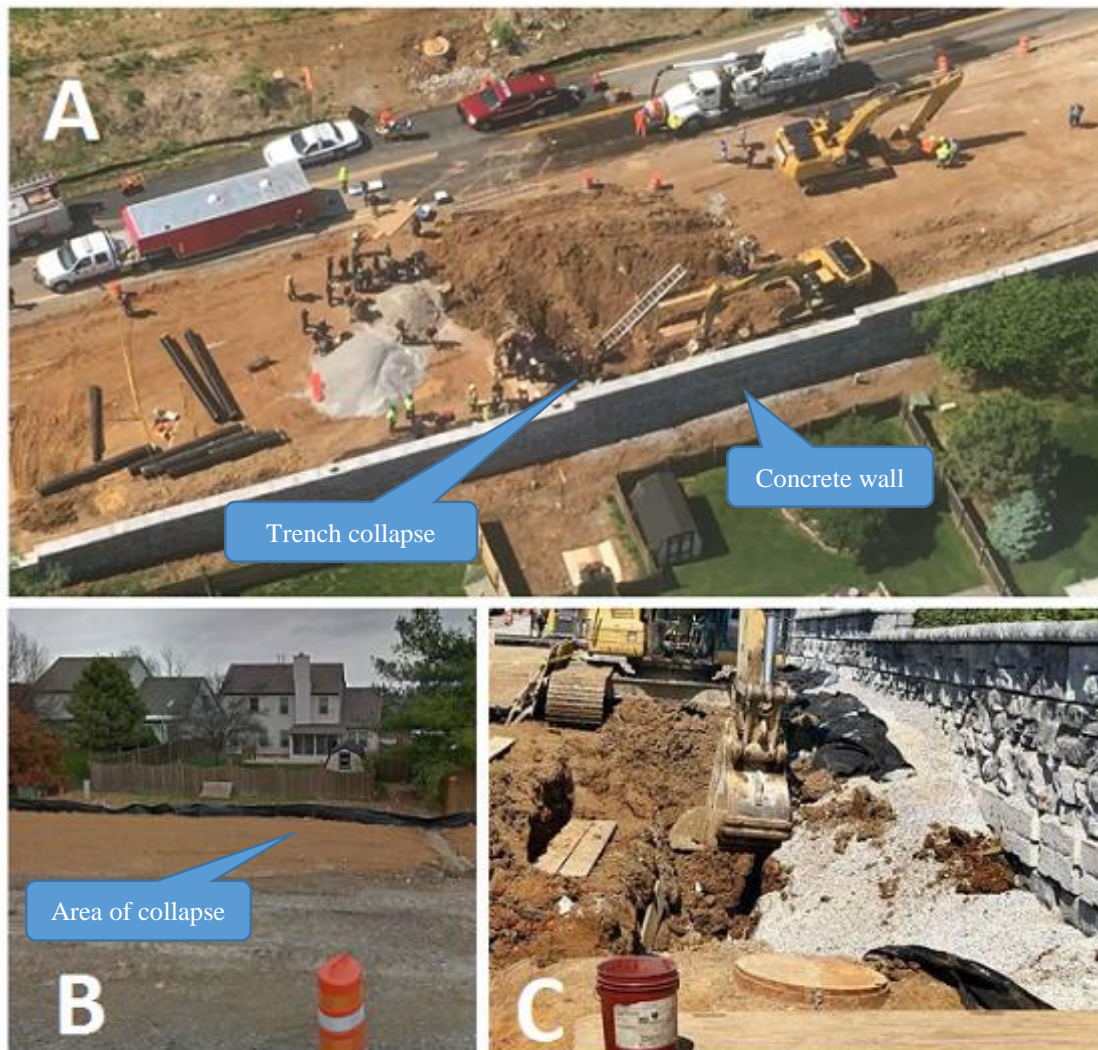
Figure 1. A) Aerial view of incident scene, B) photo of trench collapse location 4 months prior to incident, C) section of trench that collapsed on victim; concrete wall.
