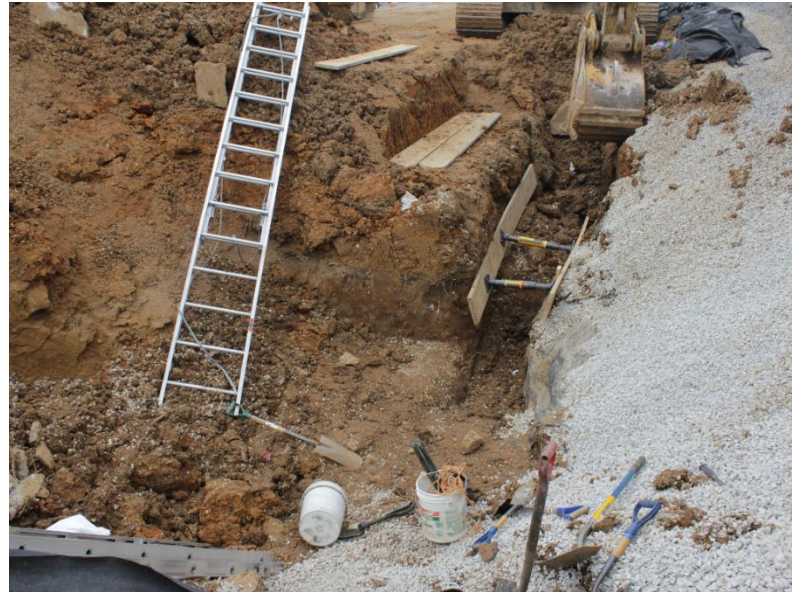
Figure 2. View looking down at the trench containing a mixture of class B and C soils on the right side of the trench near the concrete wall. Class B soil is observed on the opposite side of the trench.
