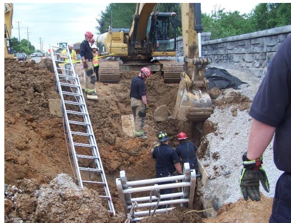
Figure 4. Trench collapse special response unit attempting to recover the victim.
