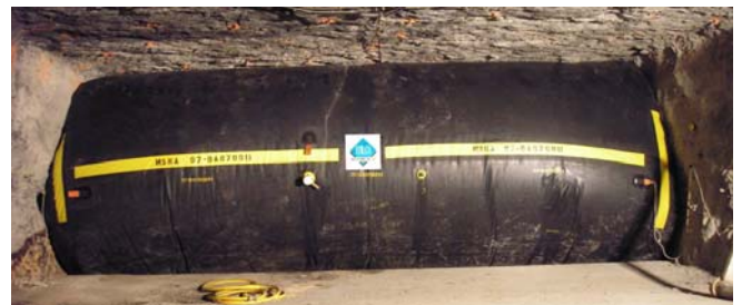
Figure 7. Fully deployed Ventsop ® unit as viewed from the C-Drift side.
