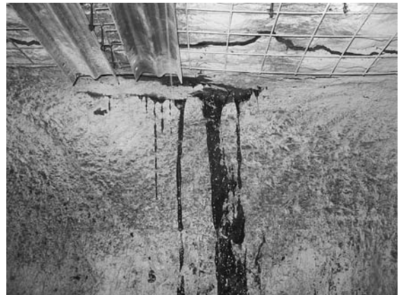
Fig. 14 PUR injected into solid roof over longwall panel migrated back to the recovery room through a cutter
