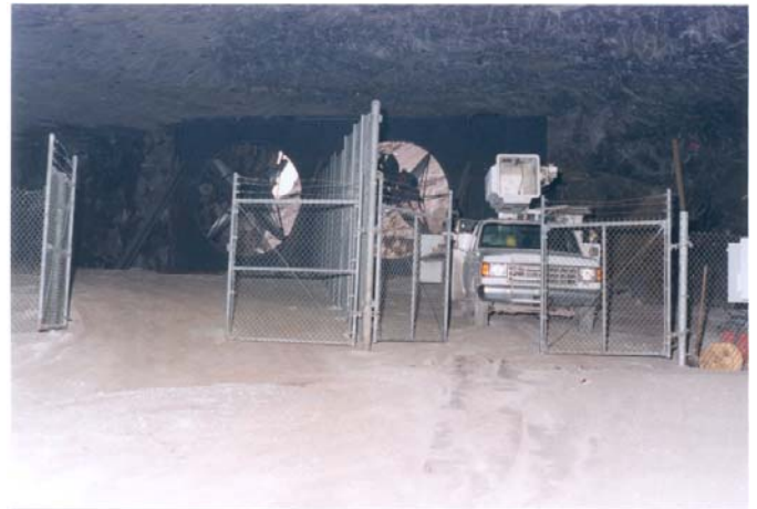
Figure 8. Fan installation with perimeter guarding during maintenance.
