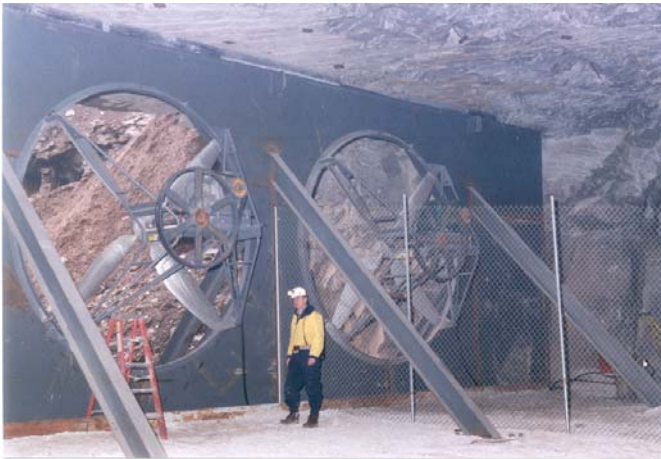
Figure 3. Two propeller fans installed for this study.
