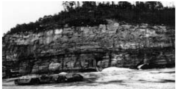
A near-vertical highwall at an Appalachian drift coal mine that poses a serious hazard to workers.
