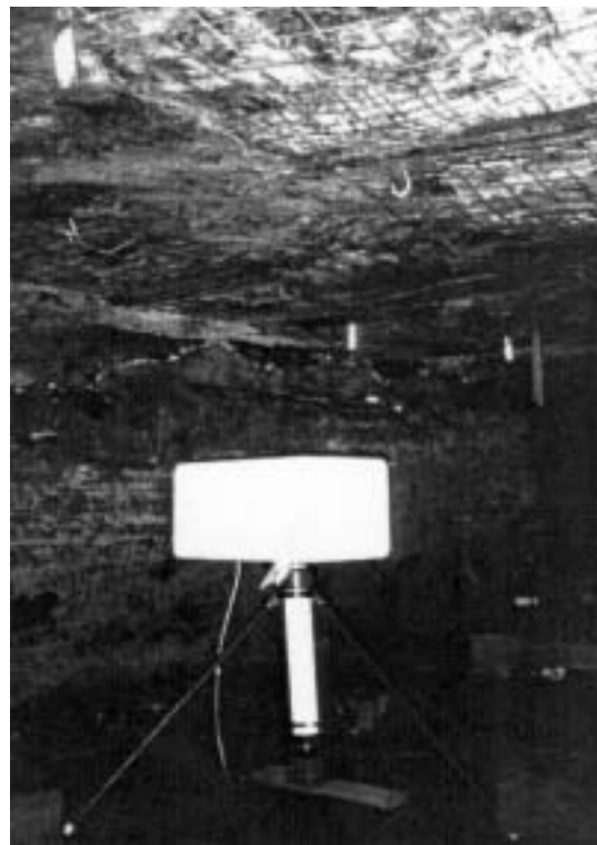
Detecting roof faults in the Bruceton mine.
