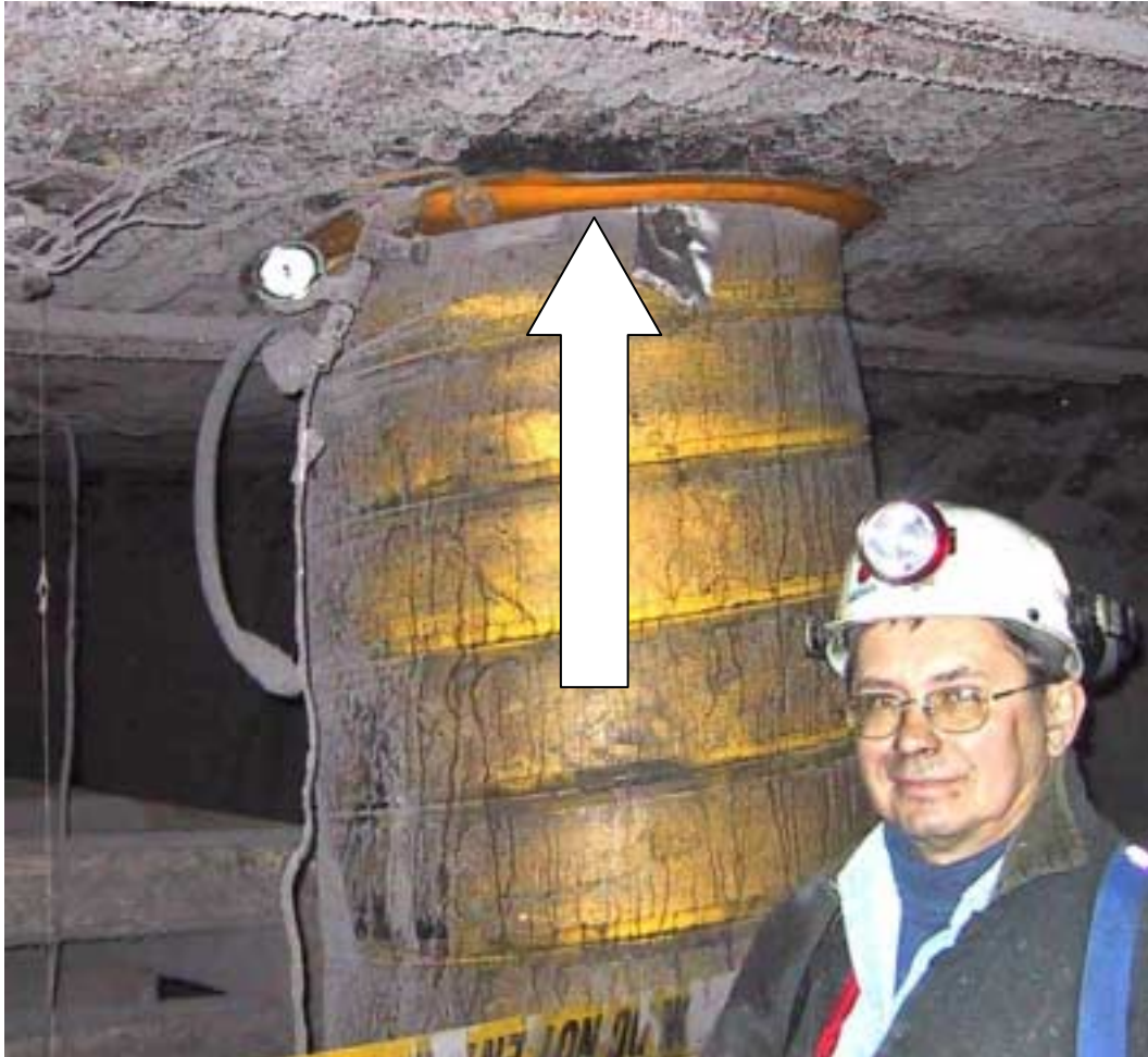
Figure 12. Hydraulic cell used to measure loading on a pumpable roof support in a longwall tailgate.
