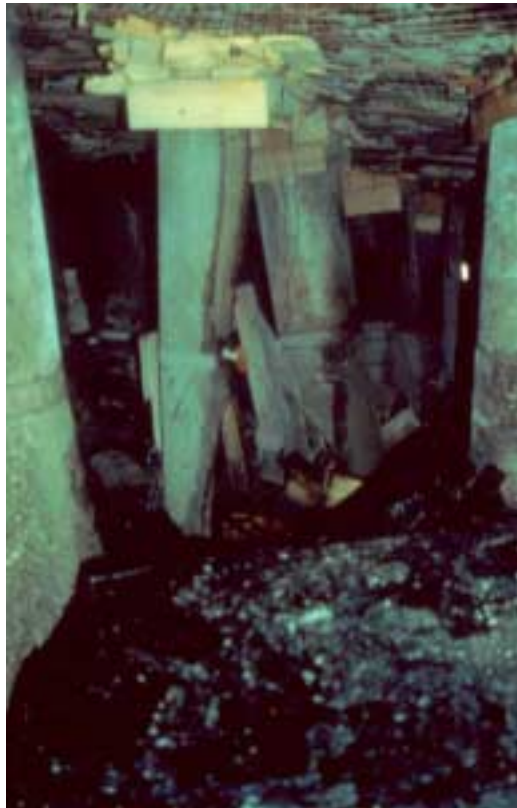
Figure 11. Failure of stiff concrete supports in a displacement-controlled environment.
