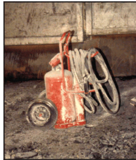
Figure 9.—Dry-chemical wheeled fire extinguisher.
