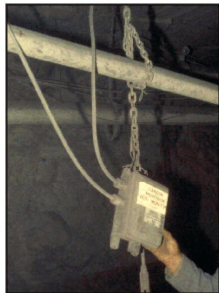
Figure 13.—CO fire sensor mounted in mine entry.
