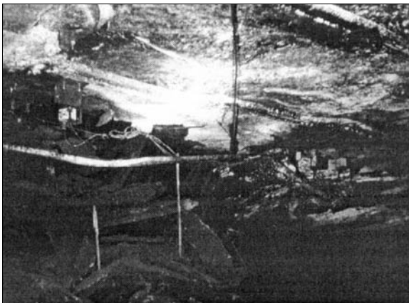
Figure 4. Photograph showing fully grouted bolts pulled from their holes in a roof fall.
