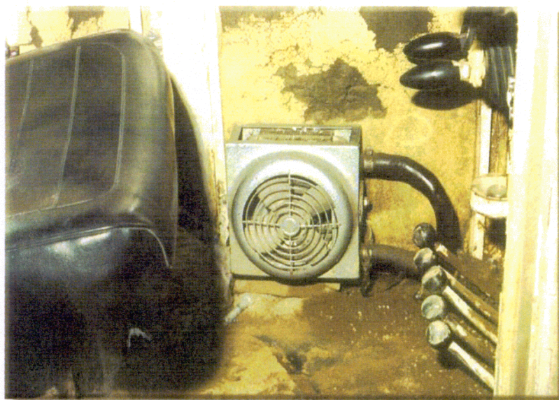
Figure 1: Location of the heater near the feet of the drill operator in the enclosed cab.
