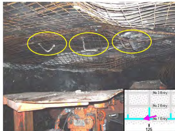
Figure 5. Damaged roof bolts in No. 1 entry after August 6 accident resulting from northern movement of southern barrier. Mesh shown was installed during rescue operations, over damaged original bolts. Camera view is indicated by arrow in index map insert (after Gates et al., 2008).
