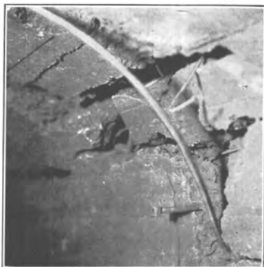
C. REINFORCING ROD PULLED OUT OF CONCRETE IN ROOF OF MAIN GALLERY.
