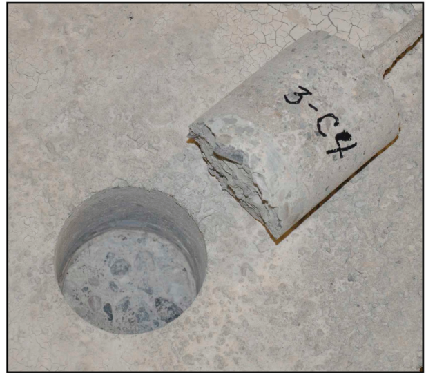
Figure 13 — Adhesion test specimen showing a tensile failure surface located predominantly in the concrete substrate.
