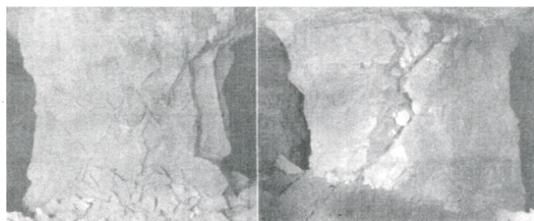
Fig. 9 Left pillar has multiple sets of discontinuities that dip at 50–70°; right pillar has two prominent discontinuities that dip at approximately 60°
