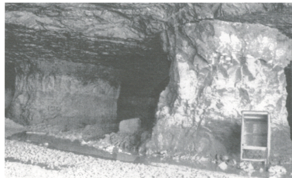
Fig. 1 Concave-shaped failing pillar. Note crushed ribs and slender appearance ( w/h < 1 ) of pillar compared with background stable pillar ( w/h > 1 )
