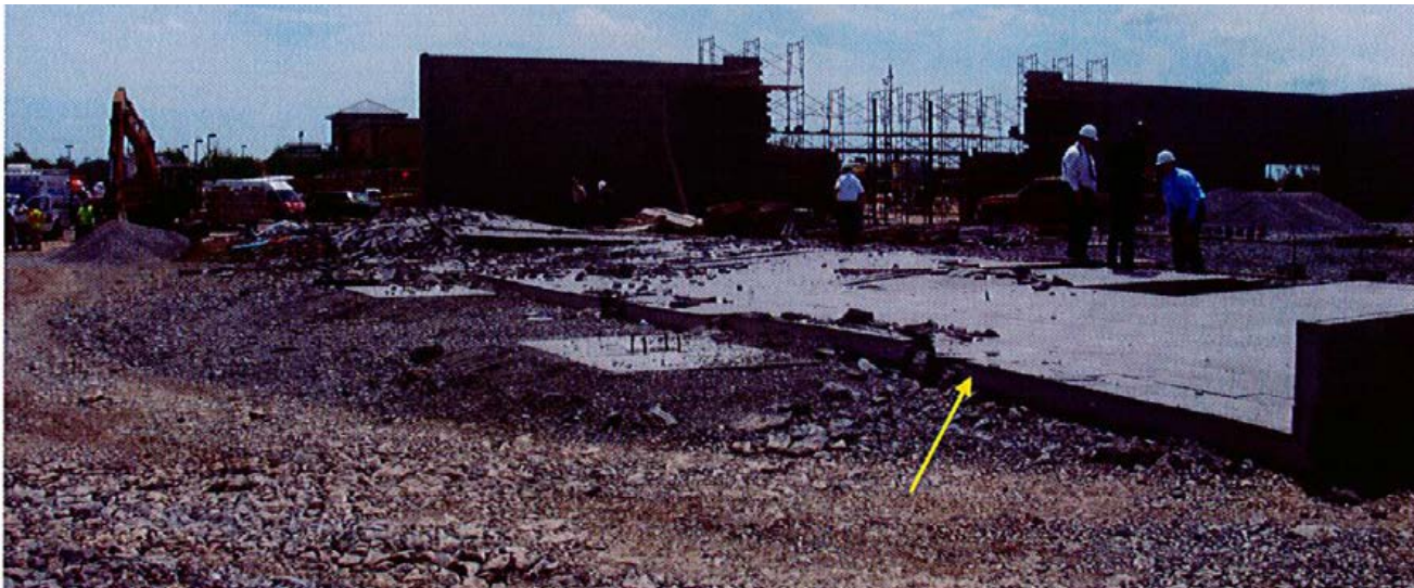
Collapsed wall (Photo courtesy of TOSHA)
