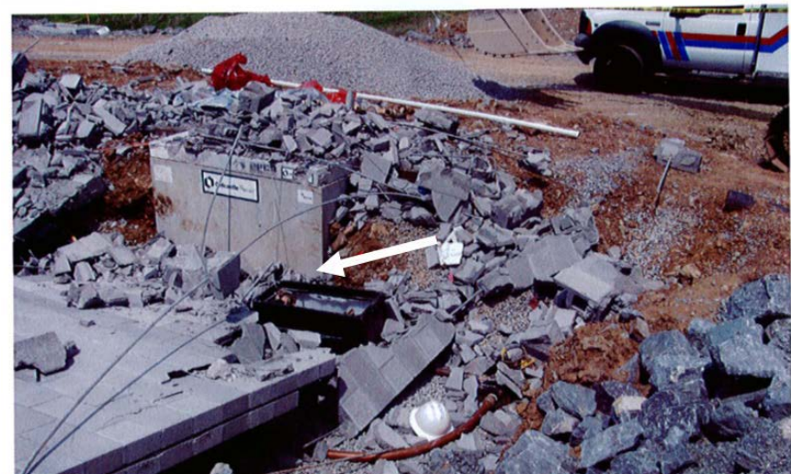
East Wall Collapsed - Arrow Indicates Location of Three Workers (Photo courtesy of TOSHA)
