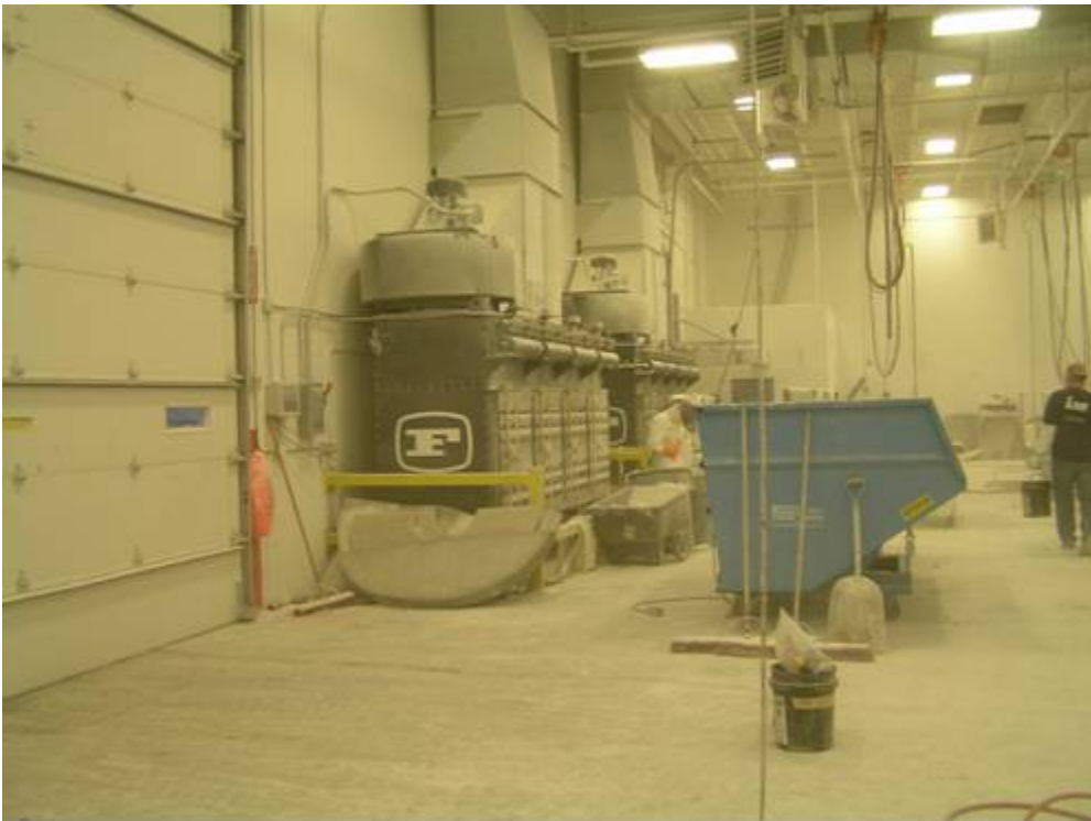
Figure 2: Exhaust ventilation in the web cut and trim area of the M Building
