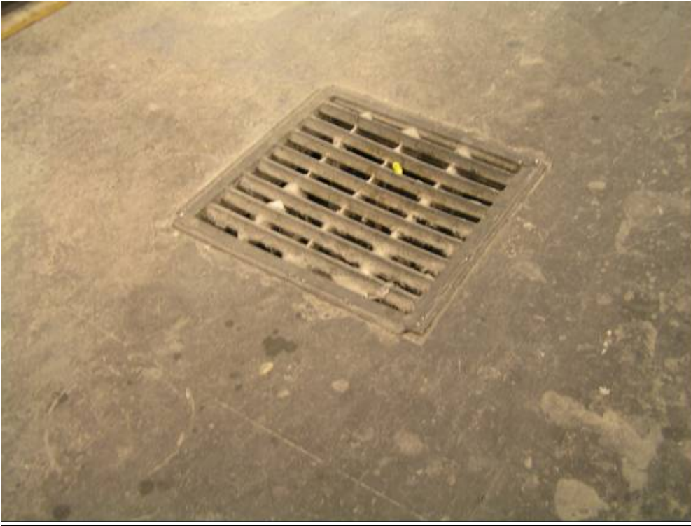
Figure 3: In-floor exhaust ventilation in the L Building
