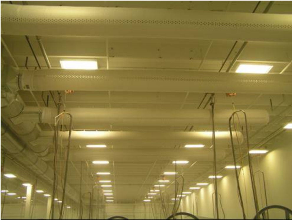
Figure 1: General ventilation supply in the M Building web cut and trim area
