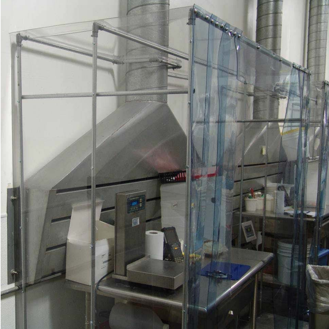
Figure 1. H2 Room ventilated work station
