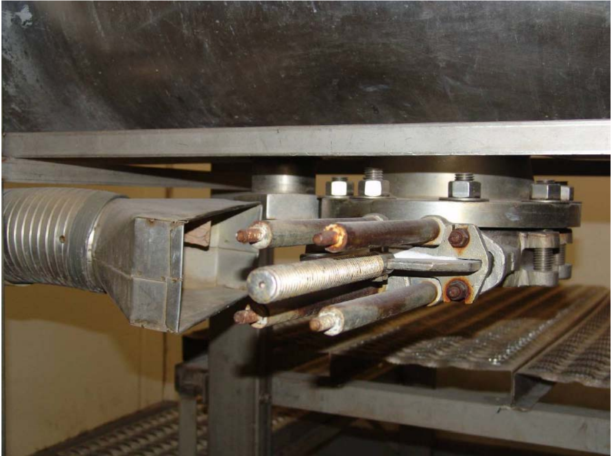
Figure 3. Blender discharge exhaust hood.
