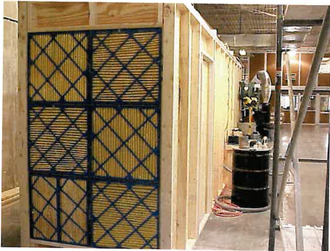
Figure 2. Photograph of the inlet filters.
