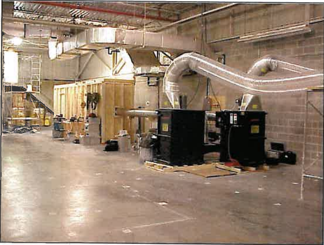
Figure 6. Photograph of the air cleaners used to move air through the test chamber. The flexible duct is set outside of the building.
