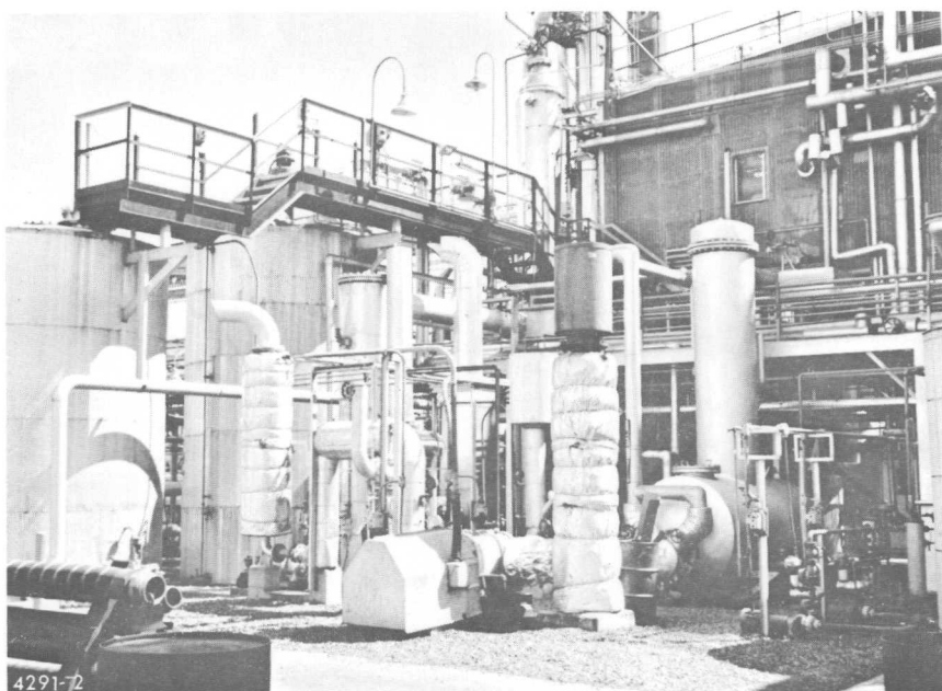
Figure 2. Enclosed reactor room in upper left hand corner. Methanol vaporizer in lower section.
