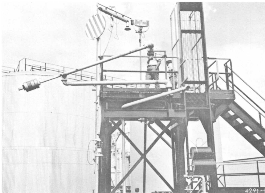
Figure 1. Methanol unloading area.
