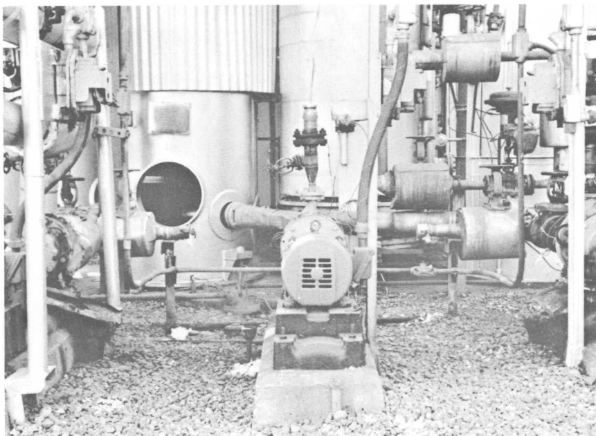
Figure 5. Spare pump from absorber.
