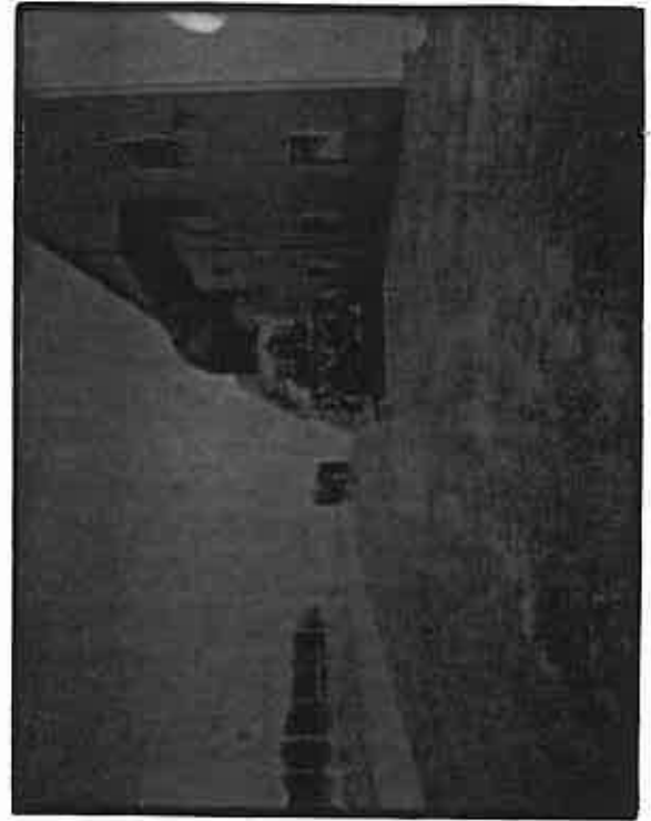
FIGURE 14. MAIN PLANT EXHAUST BLOWERS ( PLANT B )
