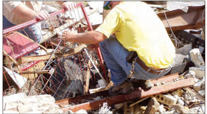
An Iowa Environmental Health Emergency Response Team member and a Louisiana Rural Water Association staff member attempt to plug a broken well head in Slidell, Louisiana, following Hurricane Katrina.
