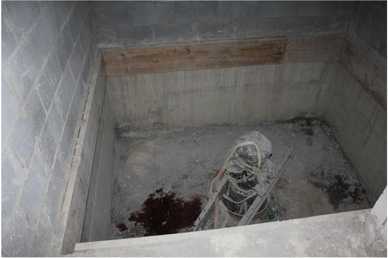
First floor landing inside elevator shaft where the victim landed. Photo courtesy of KY OSH
