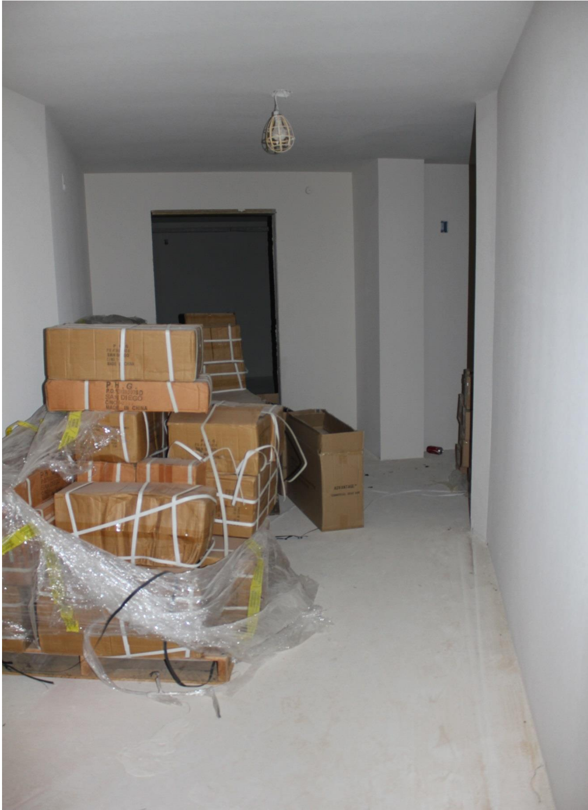
Pallets and boxes cluttering the hallway work area.
