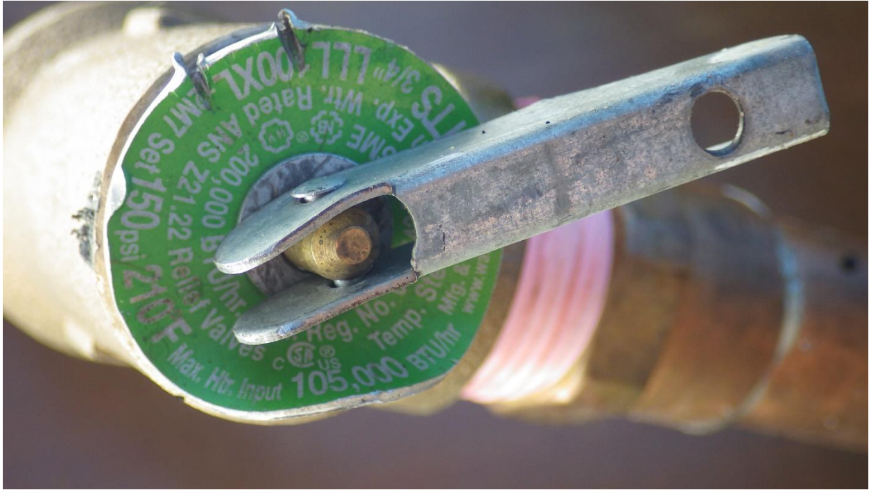
Photo #3: The PSI of the temperature and pressure relief valve. (Photo courtesy of State Fire Marshall)
