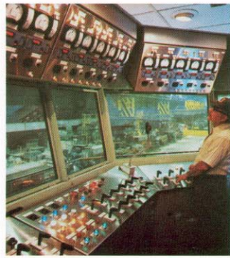
Entire rolling operation is supervised from mill pulpit , the main monitor and control center of the mill.
