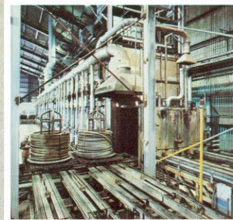
Coil annealing furnace and support equipment can handle a continuous flow of heavyweight 5400-lb coils.
