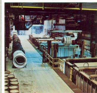
Coils as large as 5400 lb can be pickled and coated at the mill.
