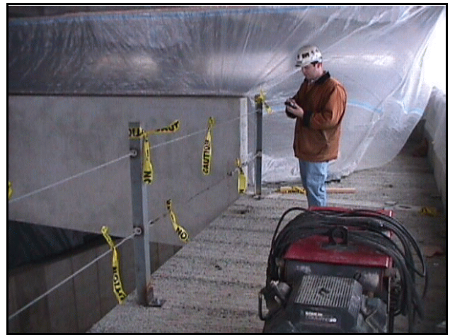
A WVU Fall-Safe coordinator audits a guard rail at a Fall-Safe contractor's site.
