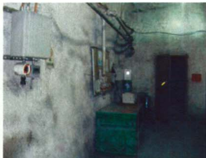
Monitoring systems, storage box
