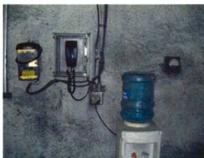
Page phone, land line, water, manometer
