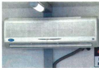
Air Conditioner Unit
